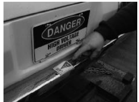
Emergency kill switch
